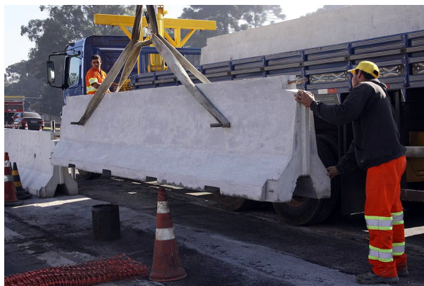
Figura 19 – Barreira New Jersey
